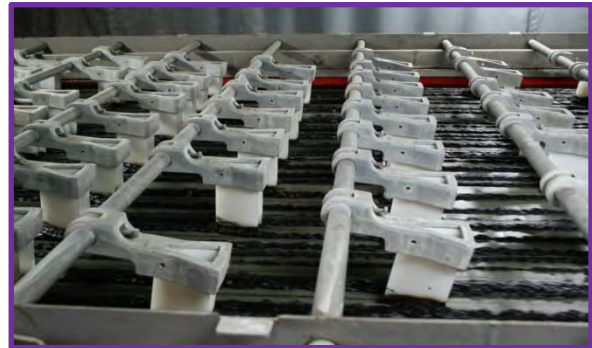
Gravity Belt Sludge Thickener
